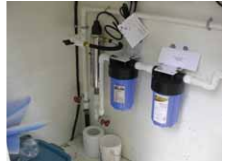
Smaller capacity sediment filters and UV light.
