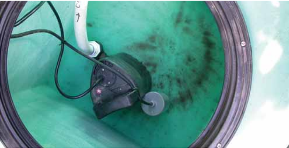
Simple pond pump in transfer tank.
