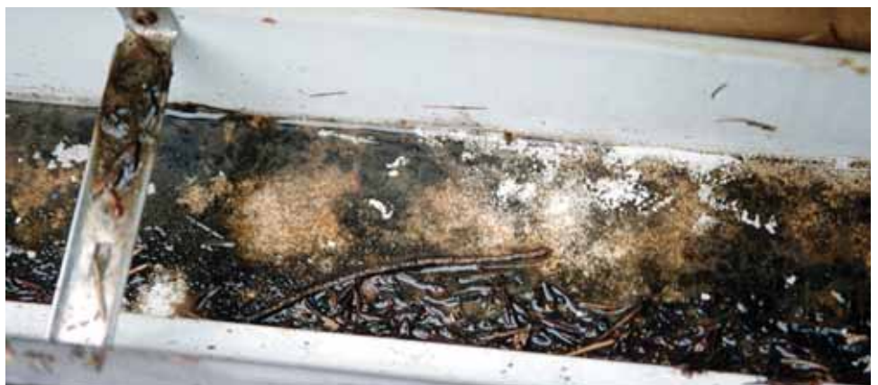
Spring pollen and debris in open gutter.
