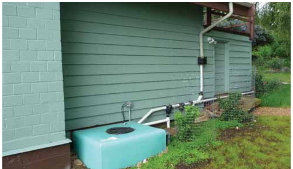
Dry triple-cleaning system to surge/pump tank, downspout to debris box, and a pair of Banjo screen mesh gravity filters.
