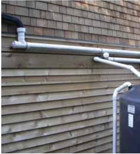
Downspouts to catchment pipe and into tank.
