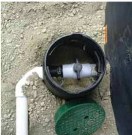
Two-inch tank exit valve.
