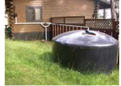
Wall-mounted pipe to 1660 gallon tank.
