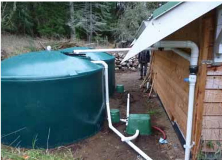
Two 1660 gal (7,550L) poly tanks with interconnecting piping and protective valve boxes (before final backfill).
