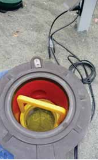
Water flowing into filter basket of whole house; combined filter and pump chamber.
