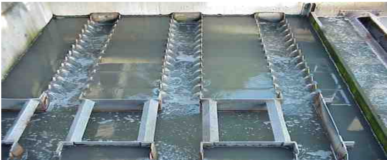
Part of the Sewage Waste Treatment Process
